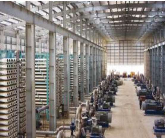
Singapore desalination plant
